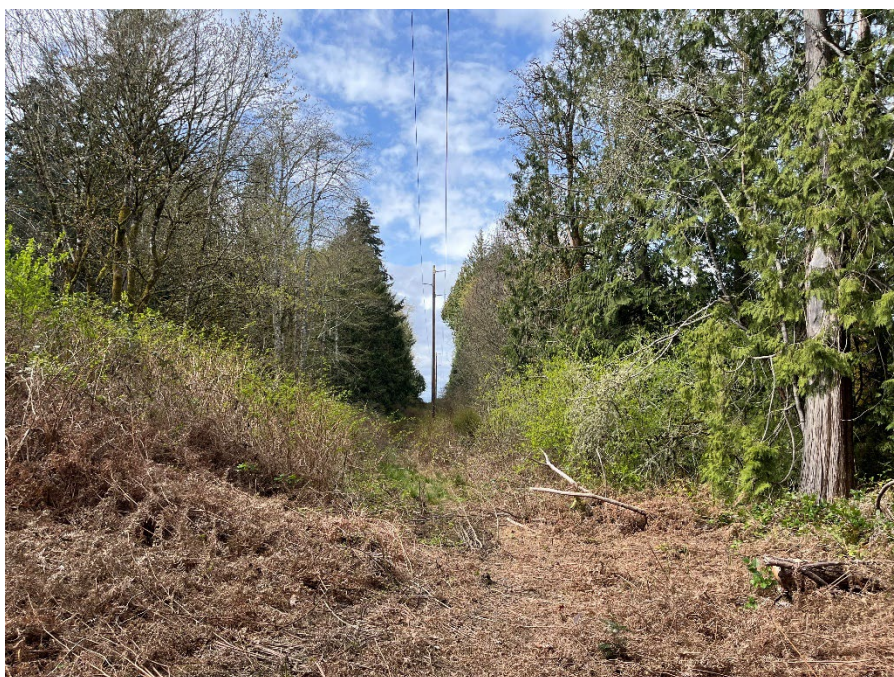
Exhibit 5. A cross country aerial transmission line viewed from Agate Pass Road NE
