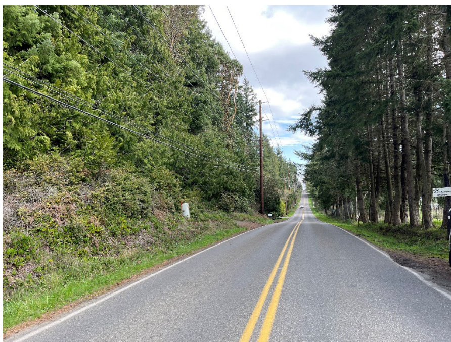
Exhibit 3. An aerial transmission line along NE Day Road
