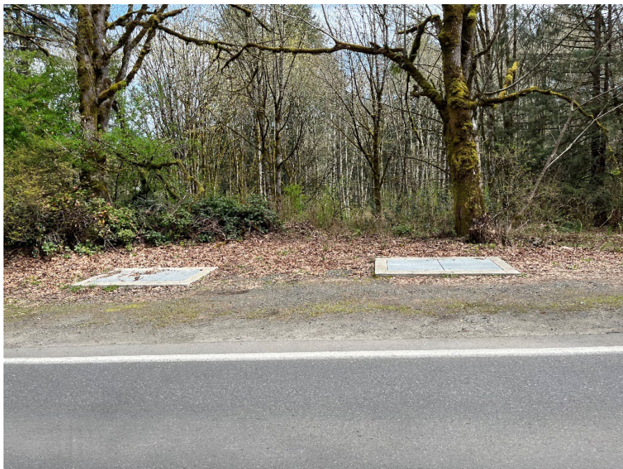
Exhibit 4. Vaults for an underground distribution line along Blakely Ave NE
