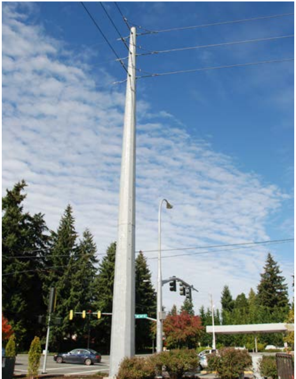
Typical 115kV Transmission Pole Steel
