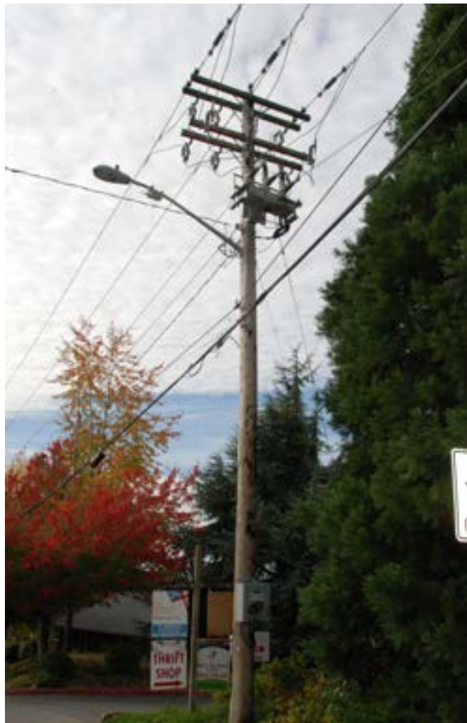
Three Phase Distribution with Recloser
