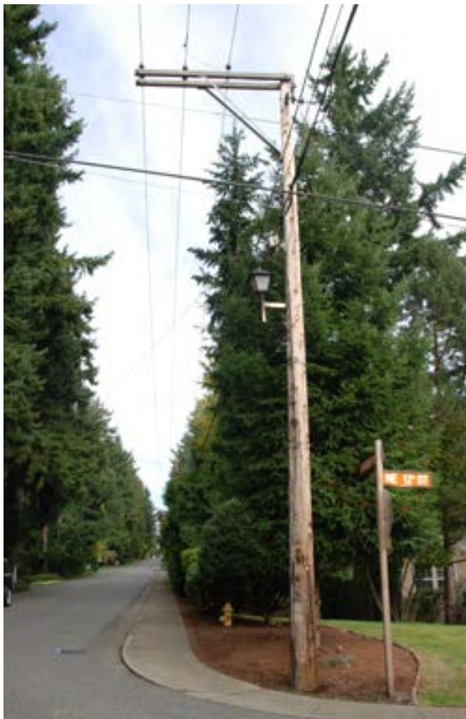
Three Phase Distribution on Wing-arm
