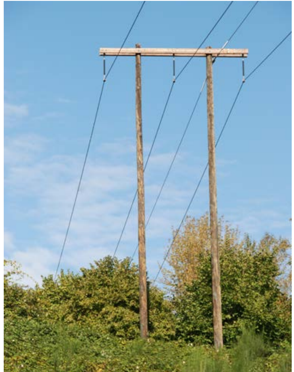
Typical 115kV Transmission H-Frame Structure
