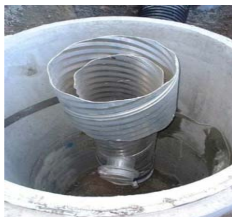
Special stormwater containment features can control water runoff roadway surfaces
