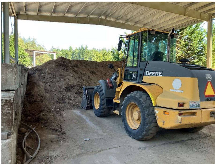
Photo [6] Description: Soil stockpile generated from road maintenance activities. Loader used to move and load soil for offsite disposal. Soil stockpiled above concrete stem wall.
