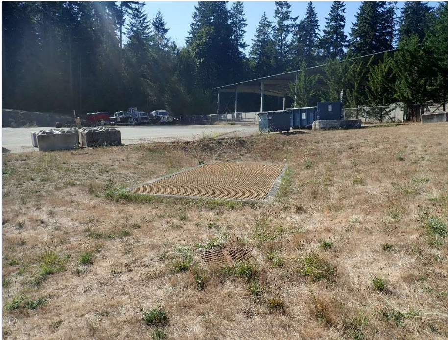
Photo [13] Description: View of sand filter and its location to decant facility.
