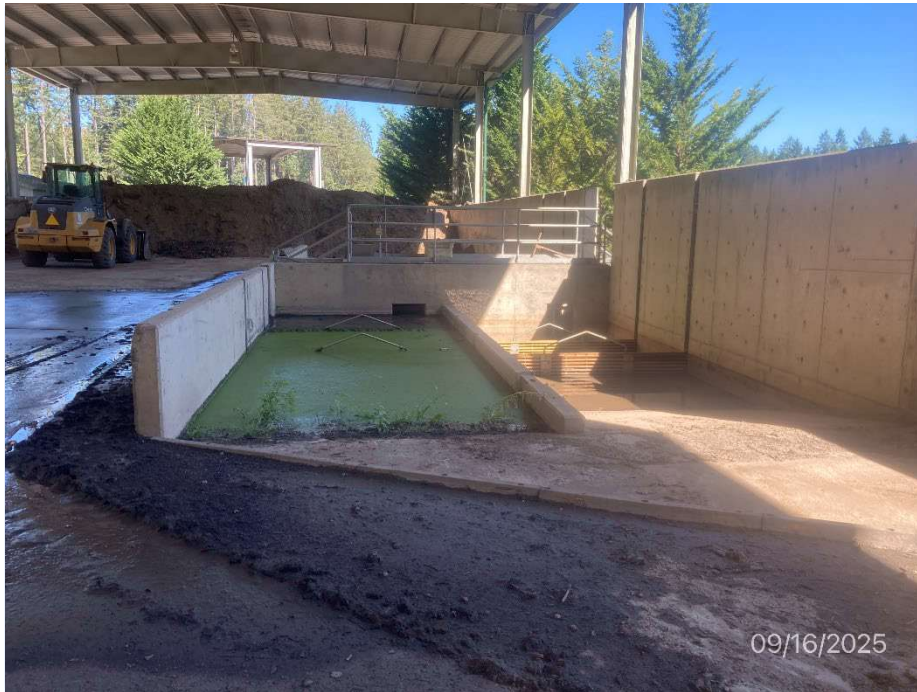
Photo [5] Description: Decant liquid settling vault, right side of the facility.
