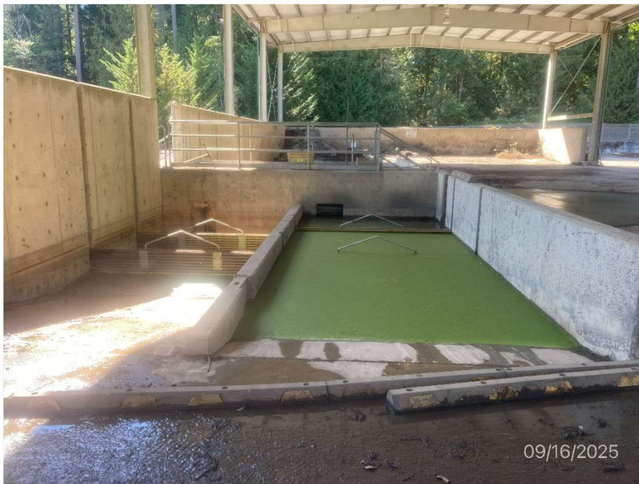
Photo [4] Description: Decant liquid settling vault, left side of the facility.
