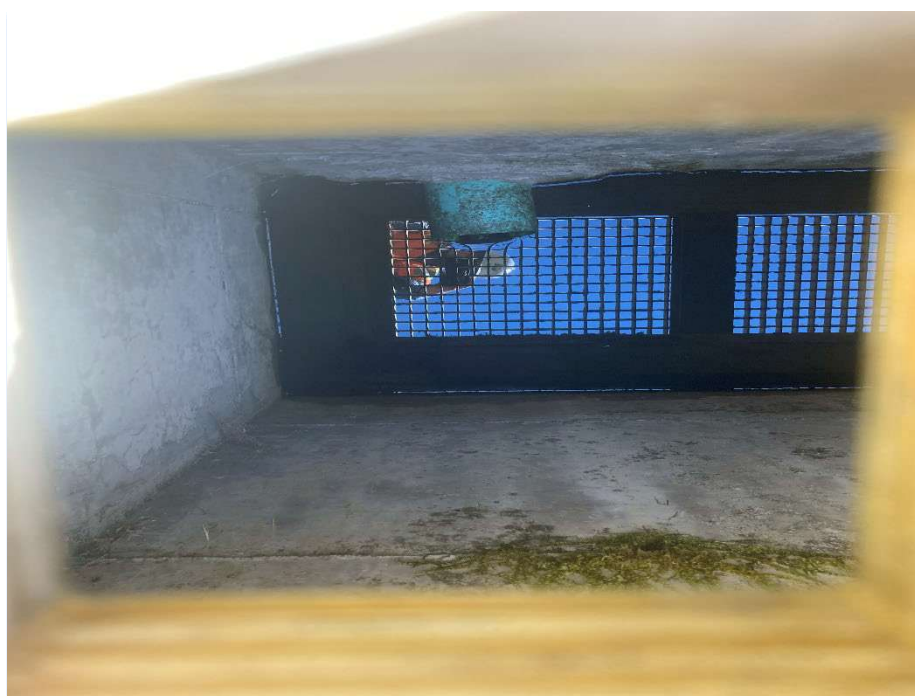
Photo [22] Description: Sand filter inundated with water.
