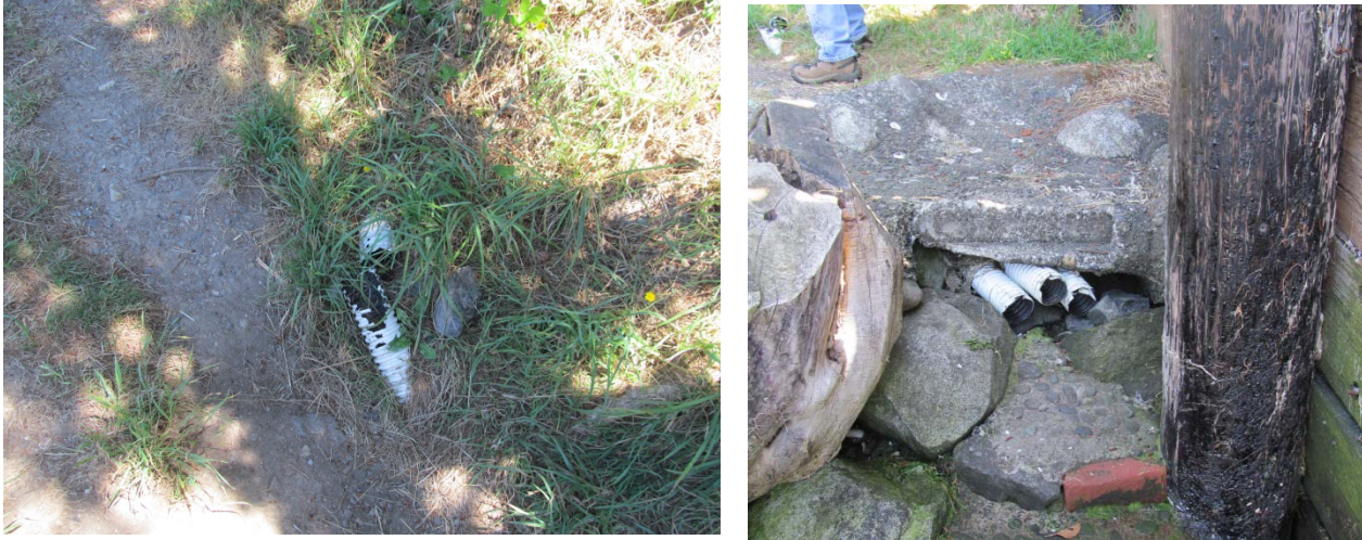
Figure 5. Broken stormwater outfall.
