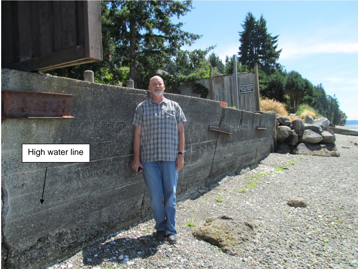
Figure 3. Visible high water line indicates highest tides/water levels approximately two feet above toe of wall.
