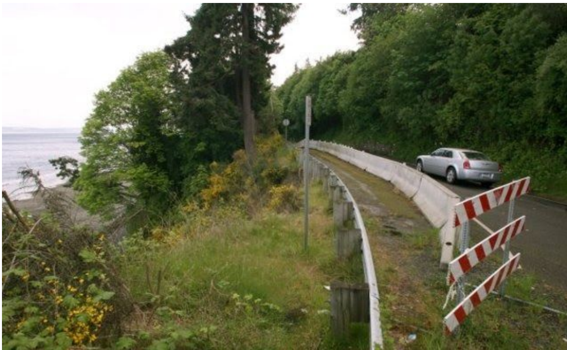
A portion of Rockaway Beach Rd. was narrowed to one lane in 2013 due to erosion. (Photo: Tad Sooter for the Kitsap Sun)
