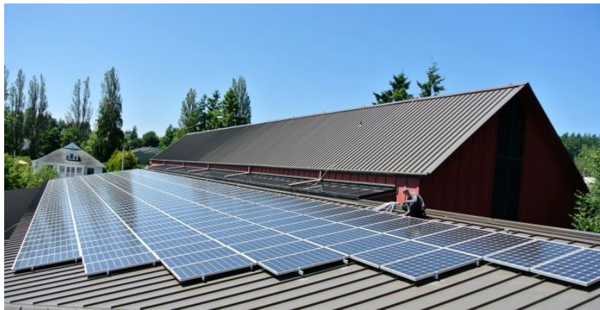
Solar panels on top of Bainbridge Island City Hall (photo: Community Solar Solutions)
