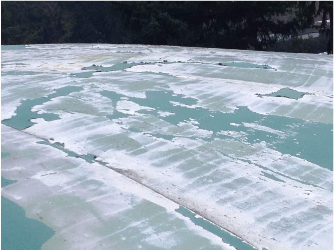
D: DELAMINATING ROOF COATING SYSTEM
