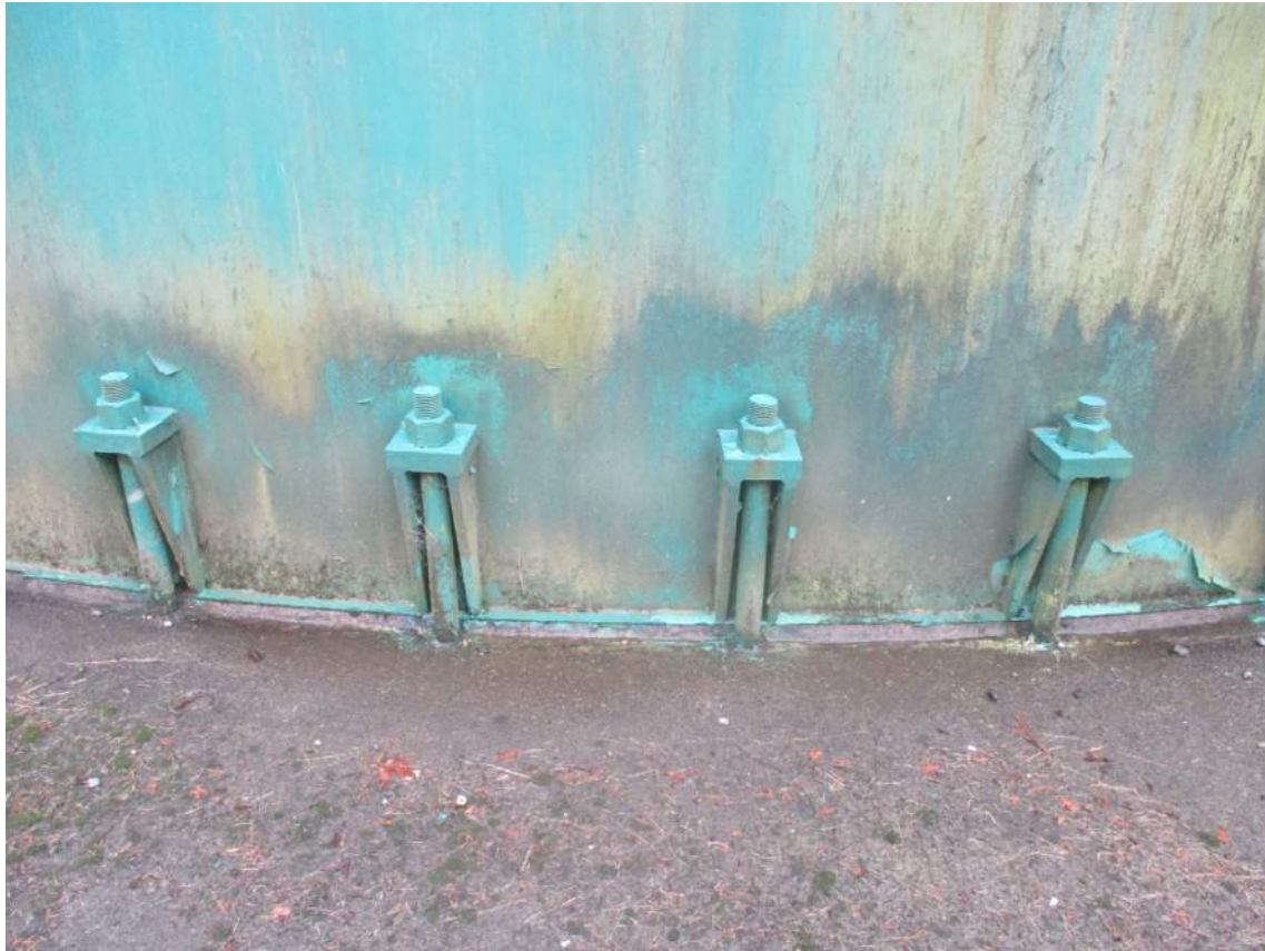
A: RESERVOIR ANCHOR BOLTS
